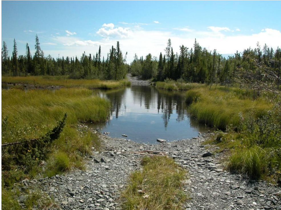
Figure 13.3: The road is flooded and may be damaged. Test the quality of the road bed by walking across before driving through water. © Bill Mitchell
