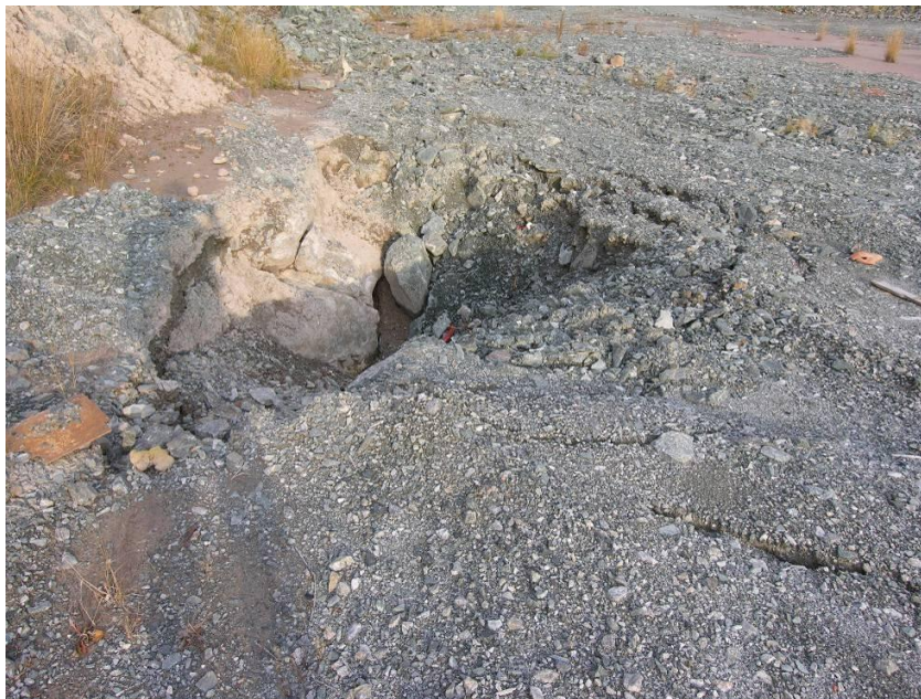
Figure 22.3: Slumping ground on the surface above underground mine workings © Courtney Mitchell
