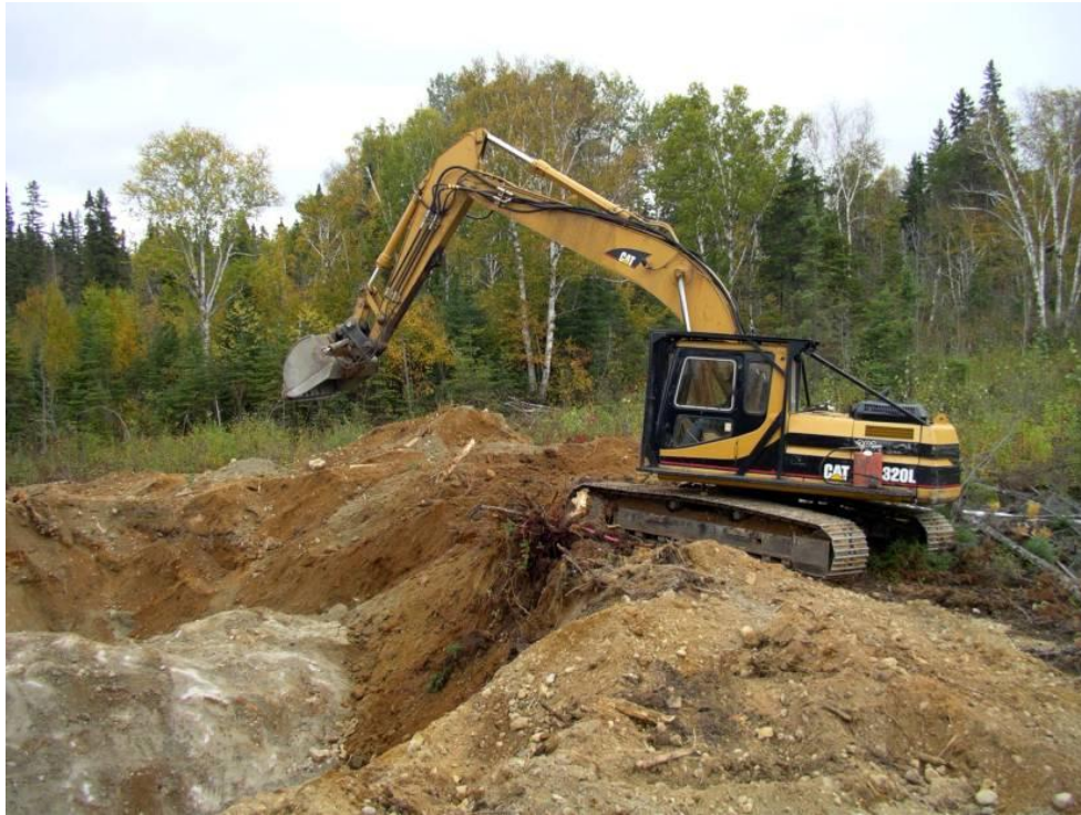
Figure 21.8: Pile the excavated material at least one metre back from the edge of the trench. © Lorne Burden
