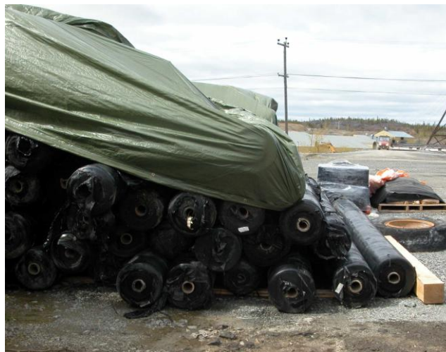
Figure 18.10: A dangerous pile of geofabric rolls: Provide adequate end support to prevent collapse. © Courtney Mitchell
