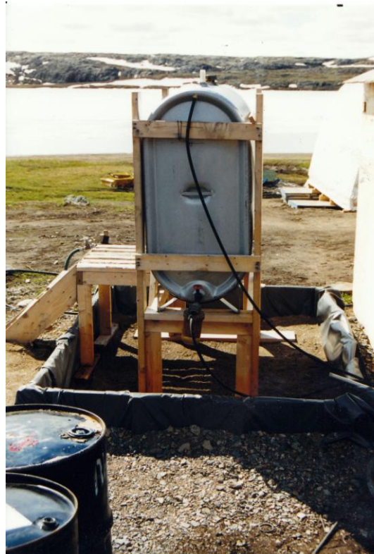
Figure 18.7: A refillable heating oil tank and berm lined with chemical resistant fabric. © Bill Mitchell
