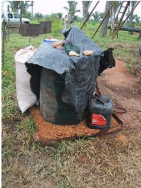
Figure 42: Drilling fluids on this project in Brazil are stored on a metal pan filled with wood chips to absorb any drips and spills. The chips can be disposed of safely at the end of the drilling. © Servitec.
