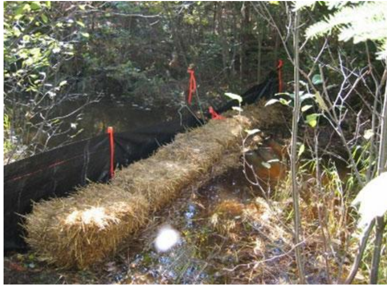
Figure 21: Used together, silt fencing and hay bales can be very effective in some circumstances. © Noranda/Falconbridge.
